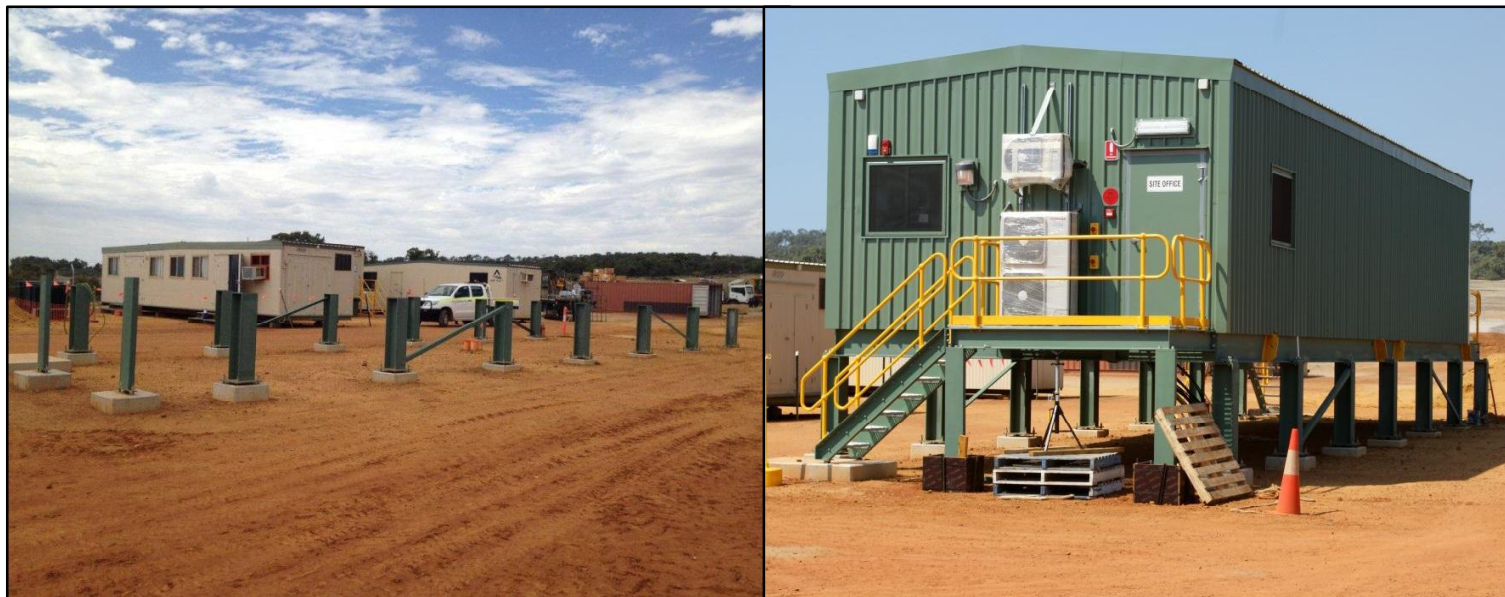
The Motor Control Centre (MCC) has been installed upon the metal bracing (left) and cabling has commenced. Final paint work to follow.
