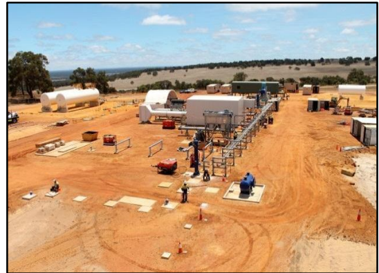
Red Gully Gas and Condensate Processing Facility, Gingin, Western Australia
