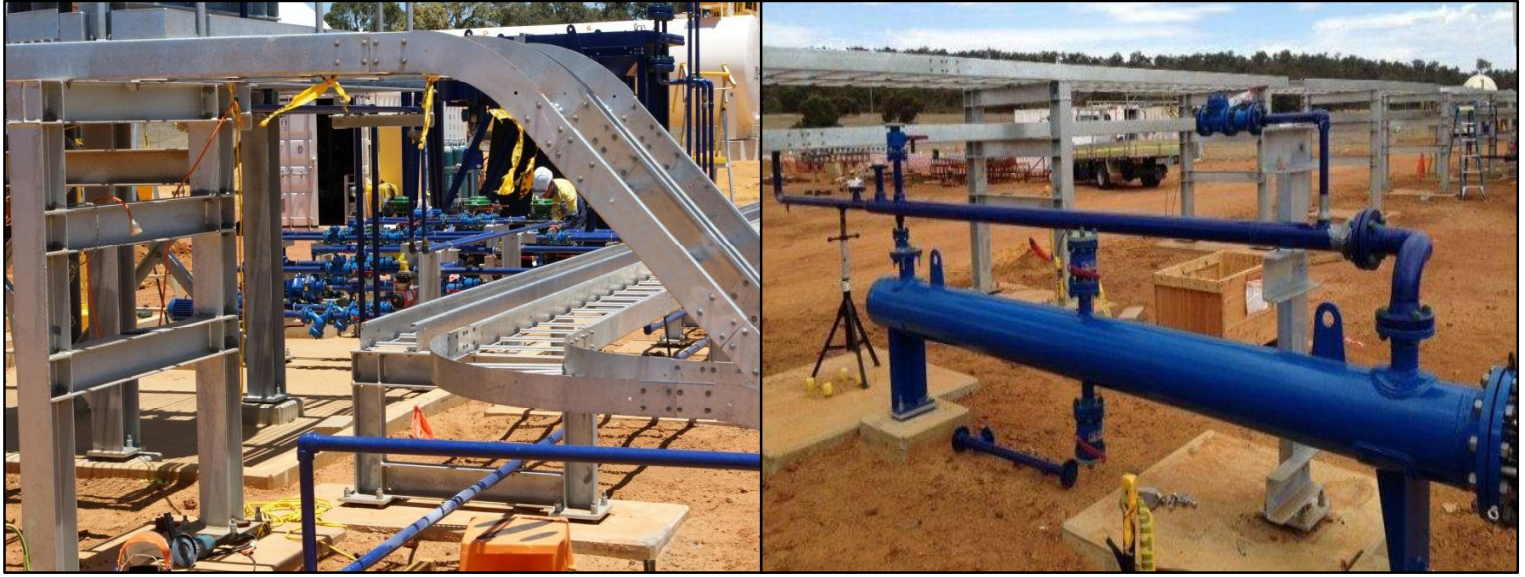
Pipework around the Facility including the Condensate Stabilisation Process Area (left) and pipework attached on the Condensate Heater (right).
