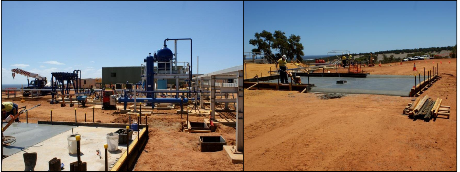
Civil works near completion in the main Facility area with concrete slabs to be poured including the Gas Metering Facility, Flash Gas Compressor and Condensate Loading Area.
