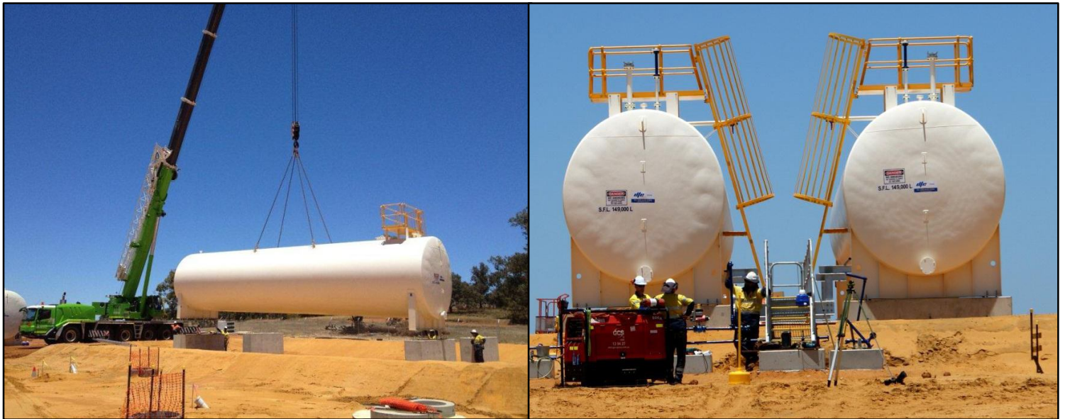
The Condensate Tanks were placed onto their supporting structure and foundations prior to Christmas. Pipe testing and gabling has been completed in early January.
