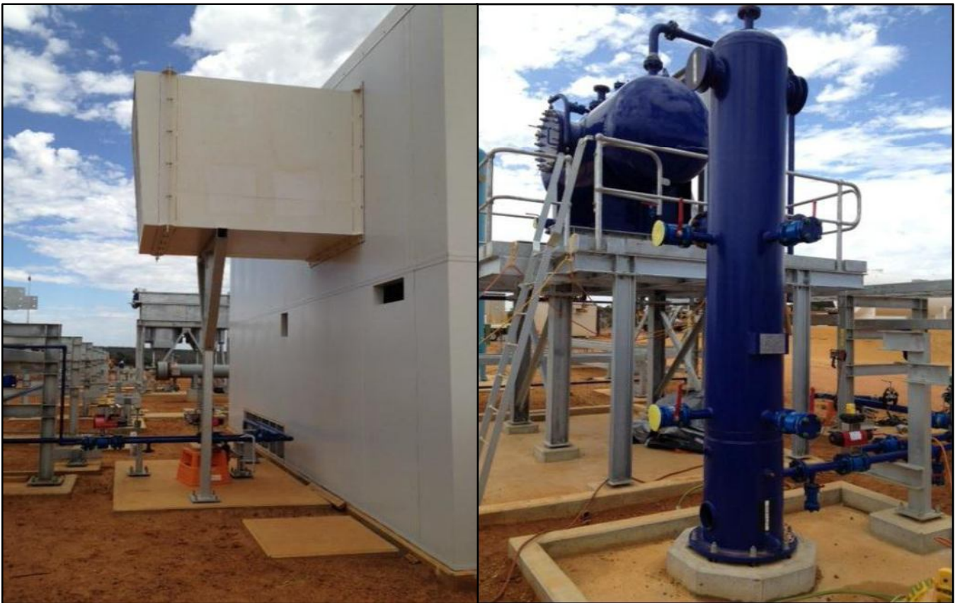
The Air Flow Vent is attached the Acoustic Enclosure (left) and Condensate Knockout Drum Valves (right).
