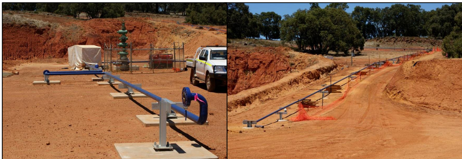
Flowline footings are being installed upon metal pipe supports from the wellhead areas towards the Facility.
